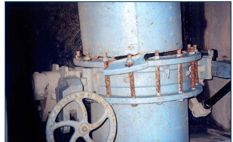
Damage to 600 mm Pipe in the Fongyuan Purification Plant
