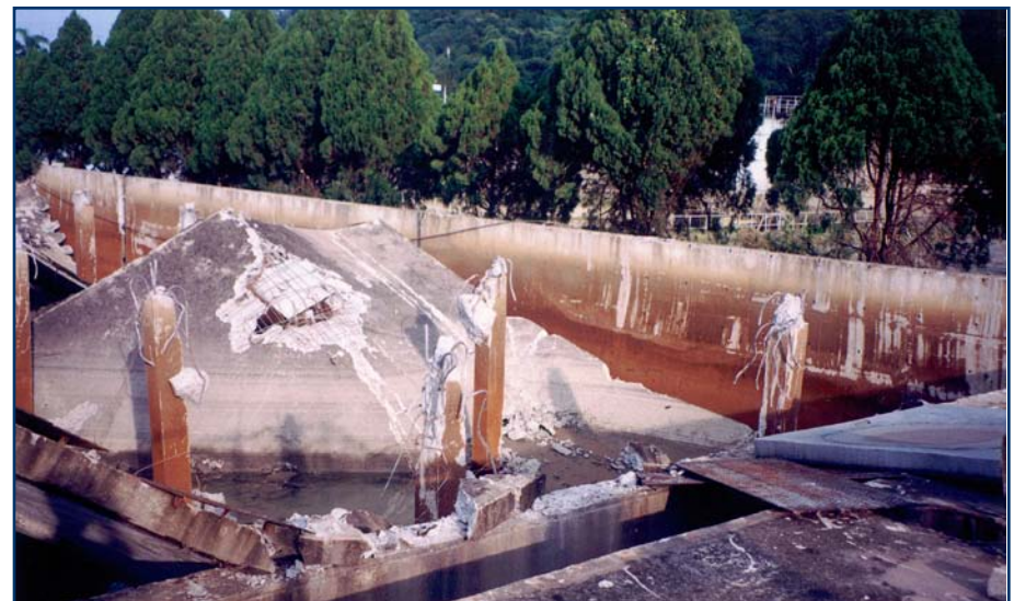
Collapse of the Finished Water Reservoir
