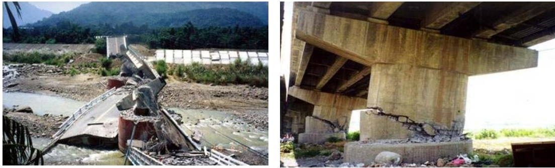
Picture 1. Damaged bridges in Chi-Chi earthquake
