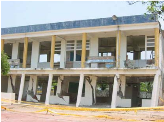
Figure 8b. RC wing wall Frame Failure
