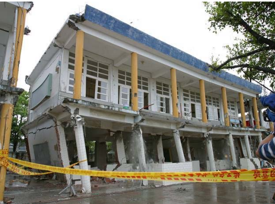
Figure 8a. Bare Frame Failure
