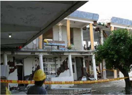
Figure 8c. Brick wing wall Frame Failure
