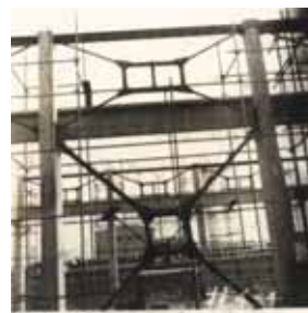
Figure 17: The 1 st structure with damper in China
