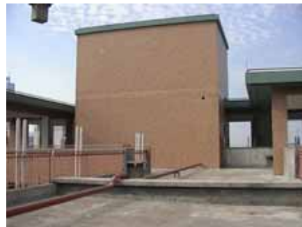
Figure 26: Water tank on top of Building
